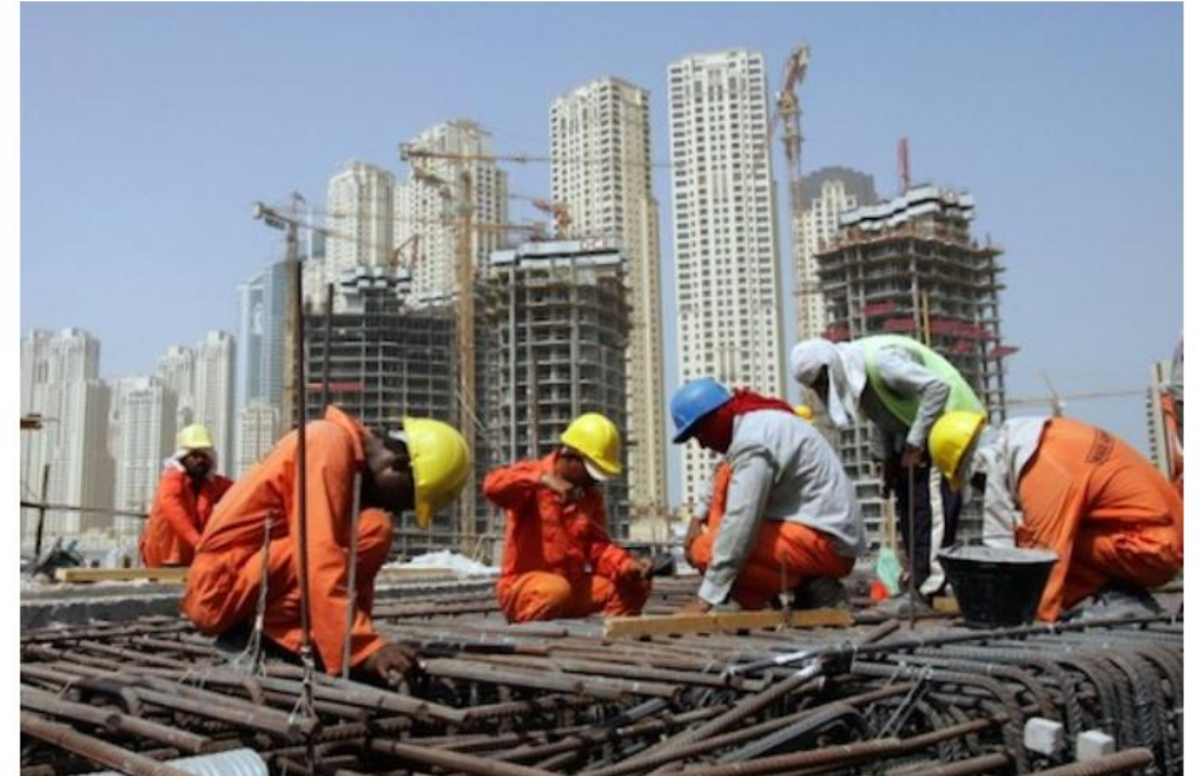
Asian workers work at a construction site in the Gulf emirate of Dubai in this file image. Dubai is one of the locations for some of Bangladesh's 10 million migrant workers who are mostly employed in the Middle East. (Photo by Karim Sahib/AFP)
